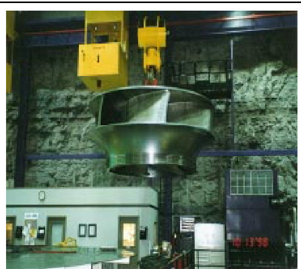
During FY 1999, ORCMT performed rapid-turnaround emergency repairs (service unavailable elsewhere) for a major Tennessee Valley Authority (TVA) facility, thus solidifying the ORCMT/TVA relationship and helping to keep Tennessee Valley electric rates from rising because of disabled equipment.
